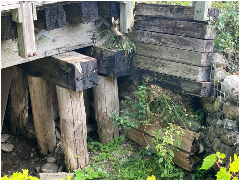
Figure 15: The southeastern ballast wall. Note the warping of the wall and vegetation growing through (A.S.I., 2024)
