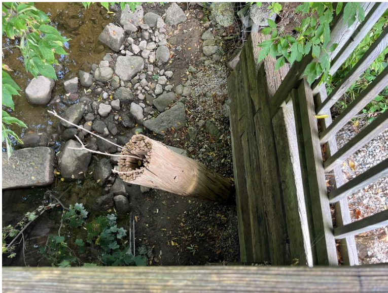
Figure 8: Detail view of the leaning northeastern ballast wall pile (A.S.I., 2024)
