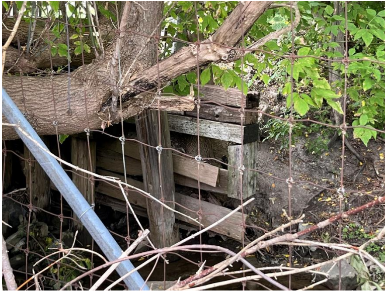
Figure 9: Detail view of the northwestern ballast wall. The tree pushing the wall inward is visible through the gap in the wall (A.S.I., 2024)
