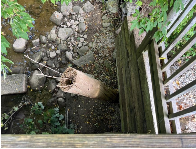
Figure 16: Detail view of the leaning northeastern ballast wall pile (A.S.I., 2024)
