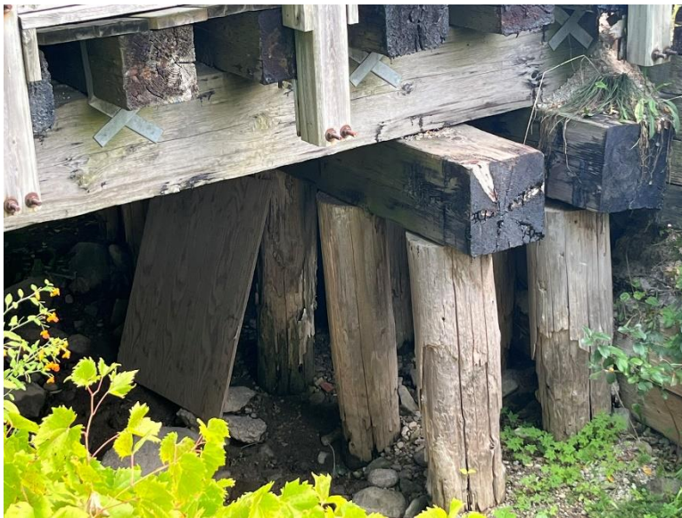
Figure 13: The bents on the eastern side of the bridge, note the leaning cap on the pier along the ballast wall (A.S.I., 2024)
