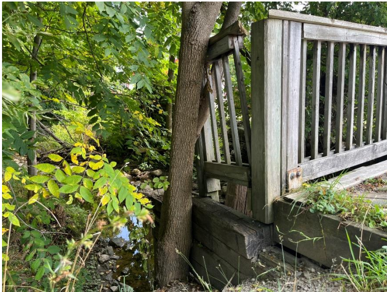
Figure 21: Detail view of the tree growing through the railing at the northwest ballast wall (A.S.I., 2024).
