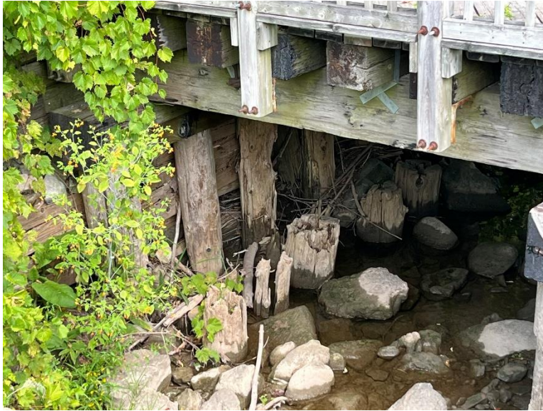
Figure 14: Detail view of the broken piles and severe deterioration on the western piers (A.S.I., 2024)
