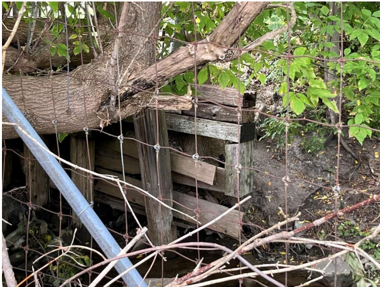
Figure 17: Detail view of the northwestern ballast wall. The tree pushing the wall inward is visible through the gap in the wall (A.S.I., 2024)
