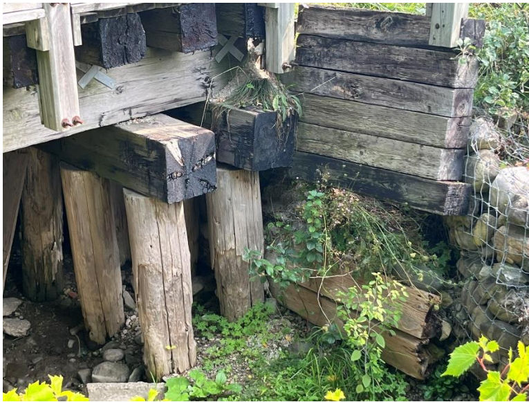
Figure 7: The southeastern ballast wall. Note the warping of the wall and vegetation growing through (A.S.I., 2024)
