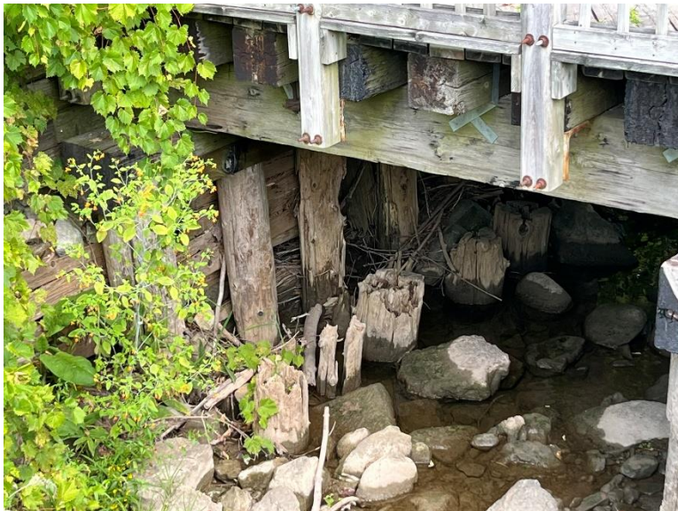
Figure 6: Detail view of the broken piles and severe deterioration on the western piers (A.S.I., 2024)
