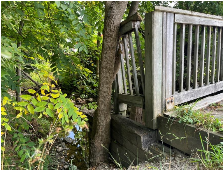
Figure 13: Detail view of the tree growing through the railing at the northwest ballast wall (A.S.I., 2024).
