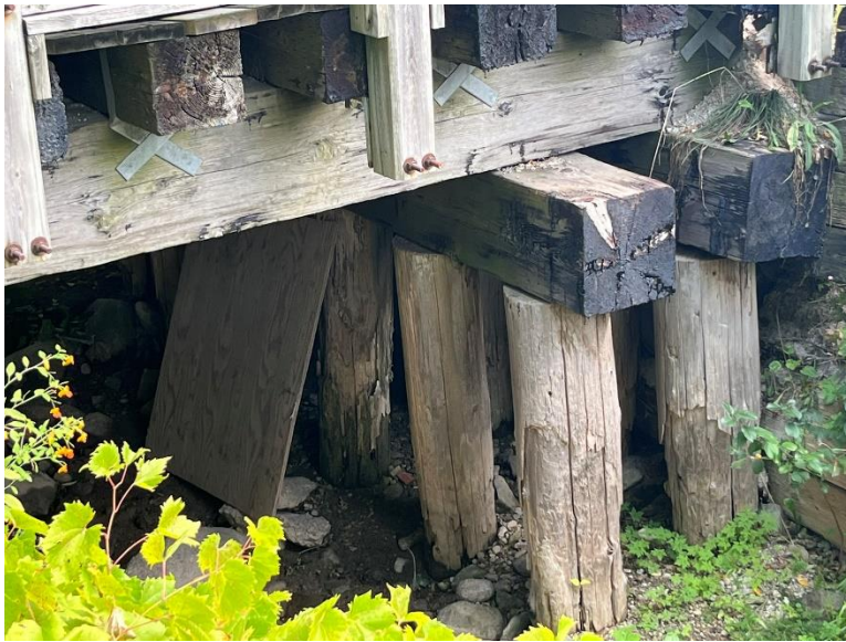
Figure 5: The bents on the eastern side of the bridge, note the leaning cap on the pier along the ballast wall (A.S.I., 2024)
